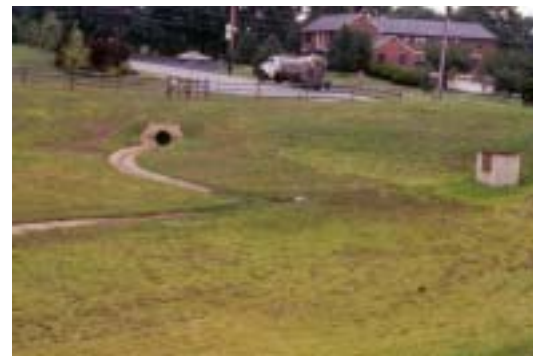
A traditional stormwater detention basin.
