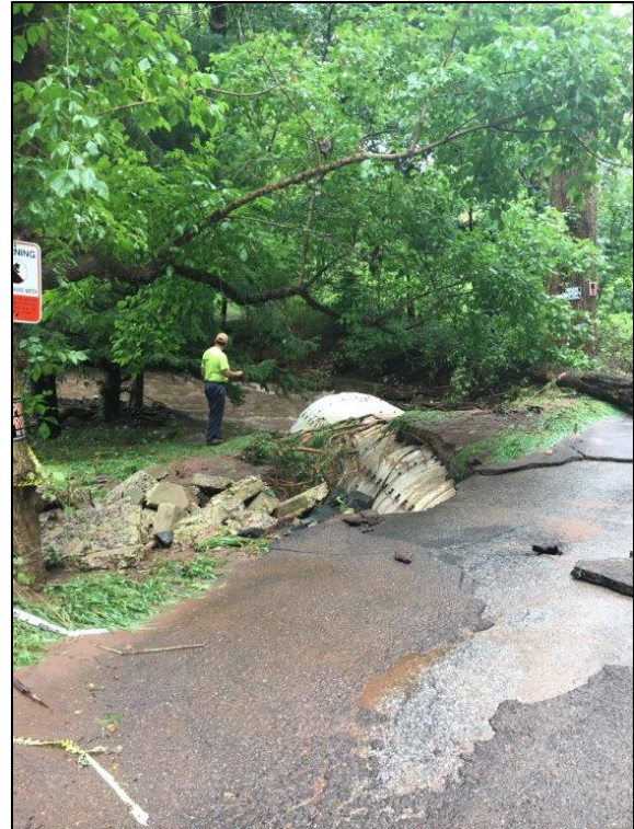
The destructive power of water is seen in this photo from October when heavy rains pulled a storm pipe out of the ground and destroyed a portion of the roadway on Catfish Lane.
